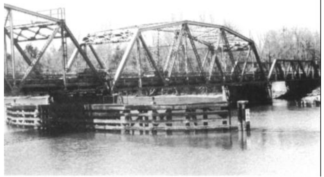
Figure 3-19. Timber bent fenders.
