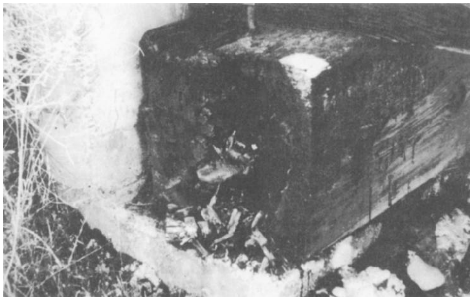
Figure 5-14. Advanced wood decay in crosstie.
